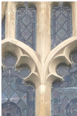
One of the north side windows showing the work done on the stone mullions.
